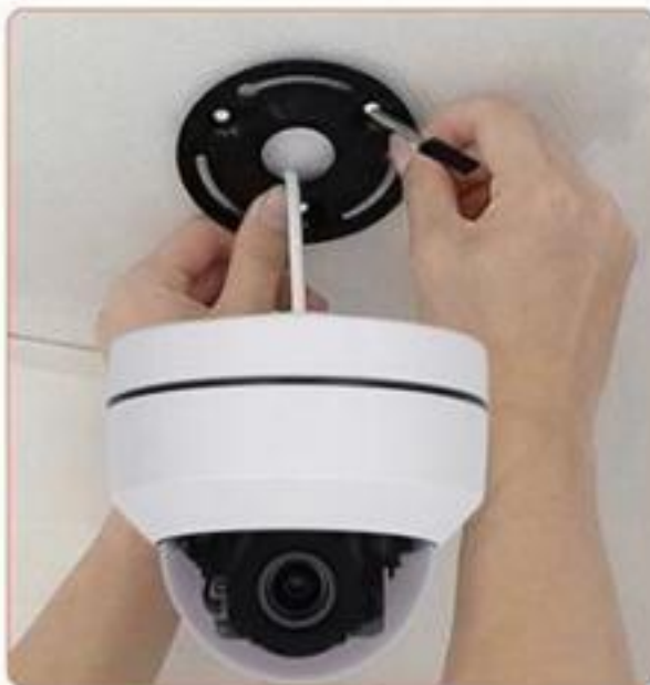
Insert the base into the tail line and lift it with the camera, then insert the screw into the expansion screw
